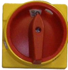
Figure 2. Primary power switch indicator
